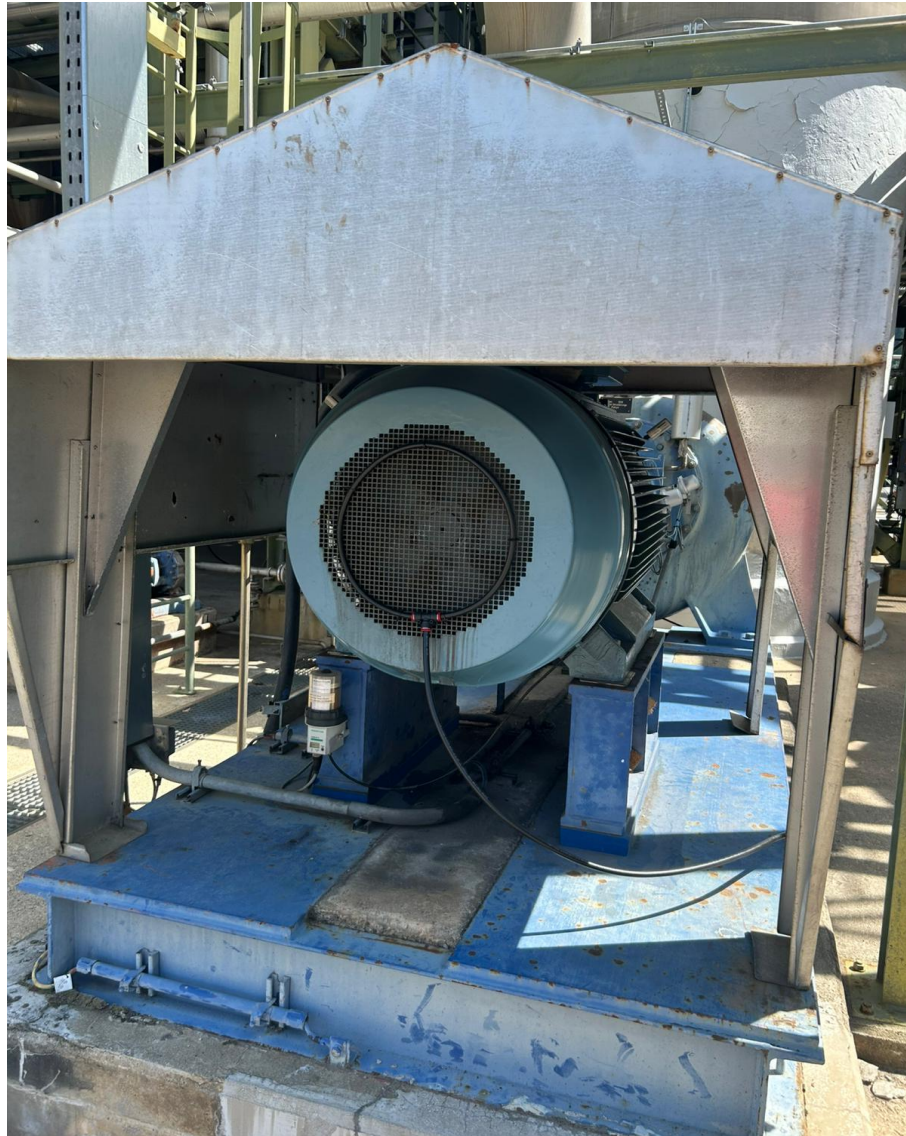
Figure 45: Engine with prior damage
