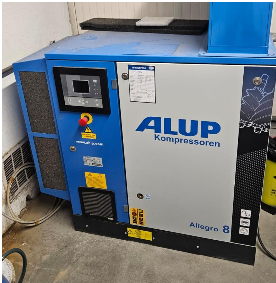
Figure 40: Monitored compressor (own illustration)
