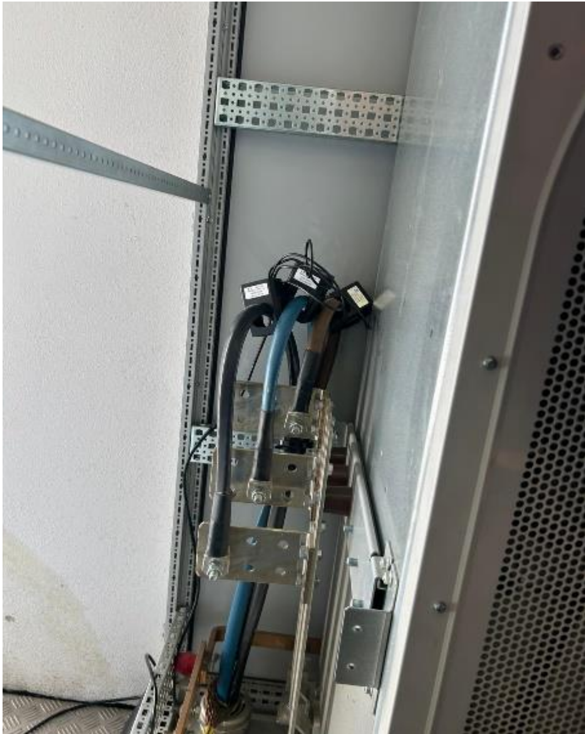
Figure 3: Installation of the current sensors (Schaeffler open source)
